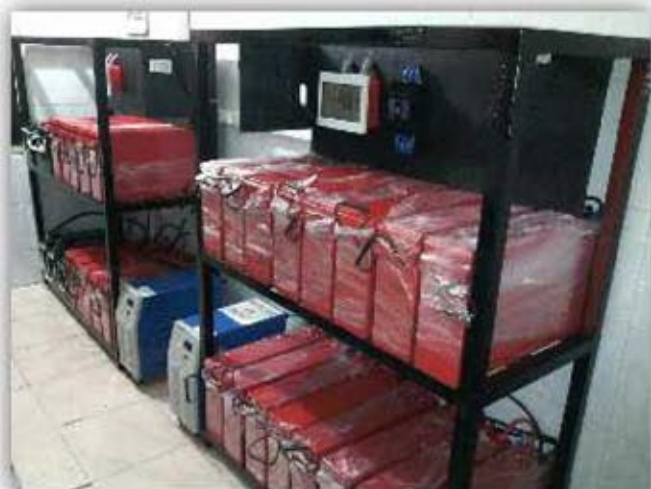
Fig.1:Community energy storage designed and installed by SMIN Power Group.
